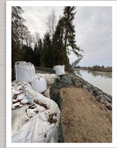
Photo 1: Damage caused by a debris strike
