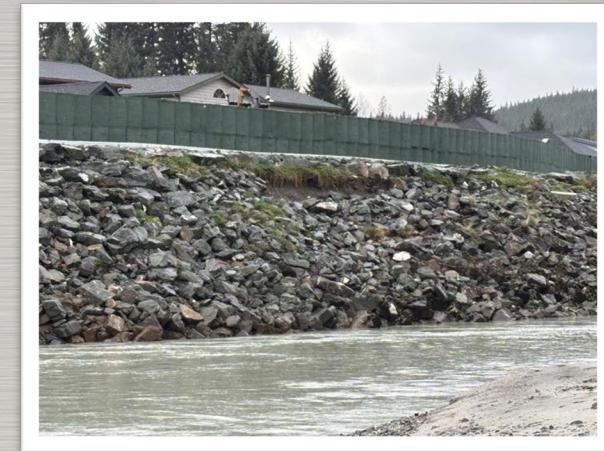
Photo 2: Slope armor sloughing down the bank
