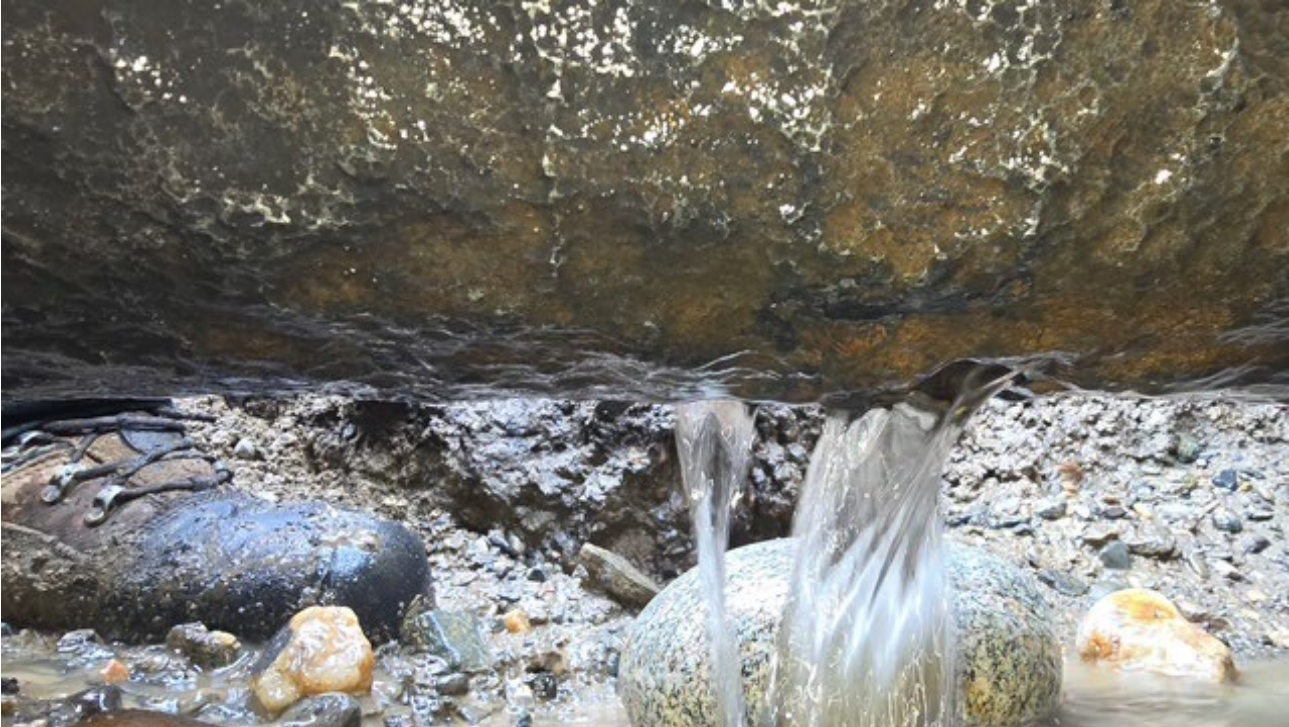
Extreme Pitting and Corrosion of Waterline and Leak
