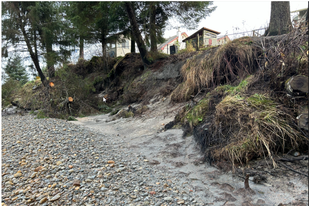
Eroding Riverbank - 3843 and 3847 Killewich – October 2024
