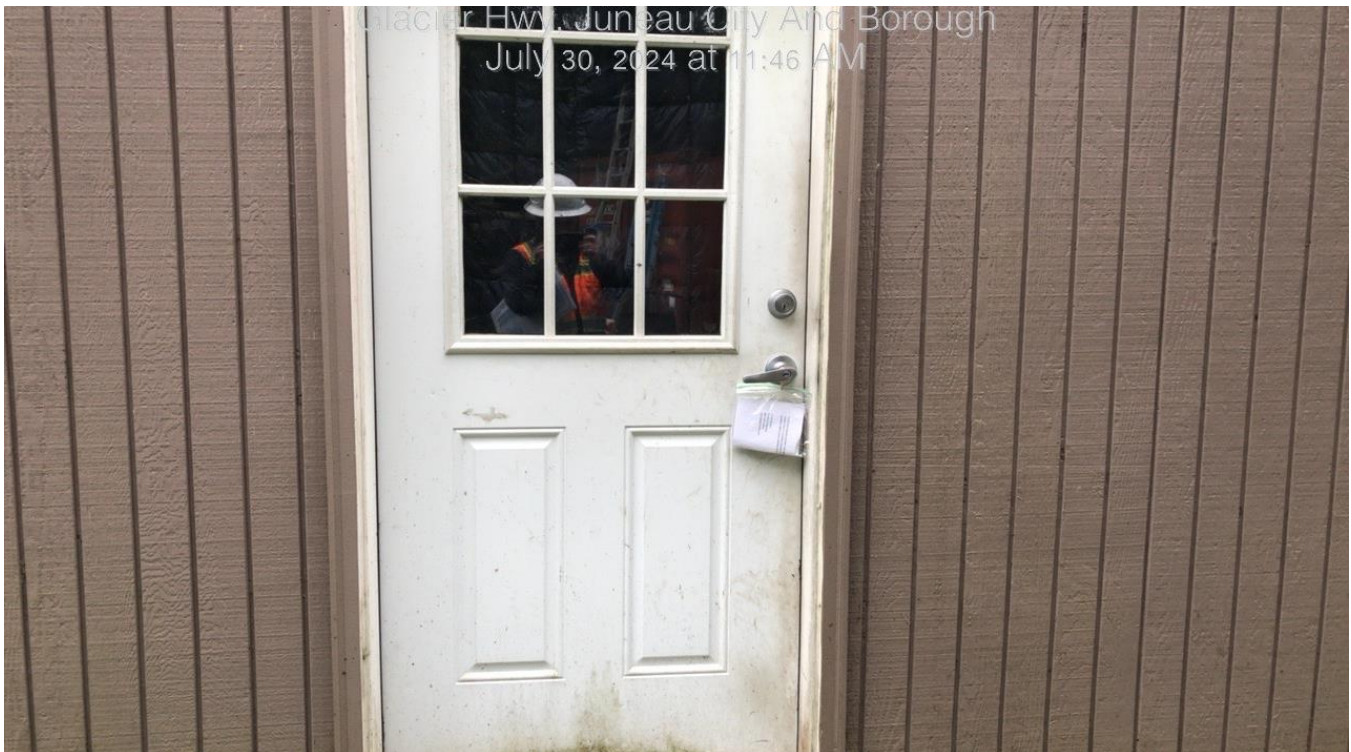
A note that was left at 16216 Glacier Hwy regarding the water service that is not currently in use.
