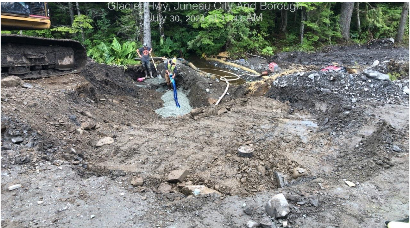
A valve box installed at the corp. stop for the water service to 16216 Glacier Hwy. This was NOT connected to the existing water service, which is currently not in use (see "Construction/Design Issues/Concerns" section for more info)
